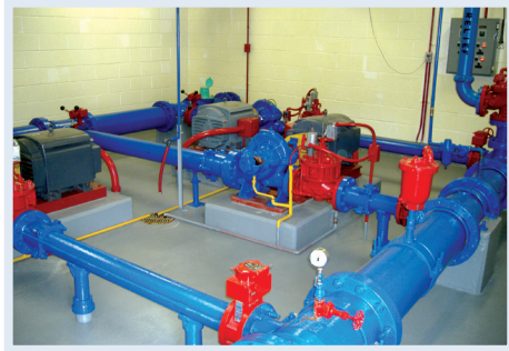
Water Treatment Plant Distribution Pumping System
